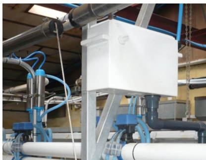
HEADER TANK (Note: Installed Level With Cylinders)
